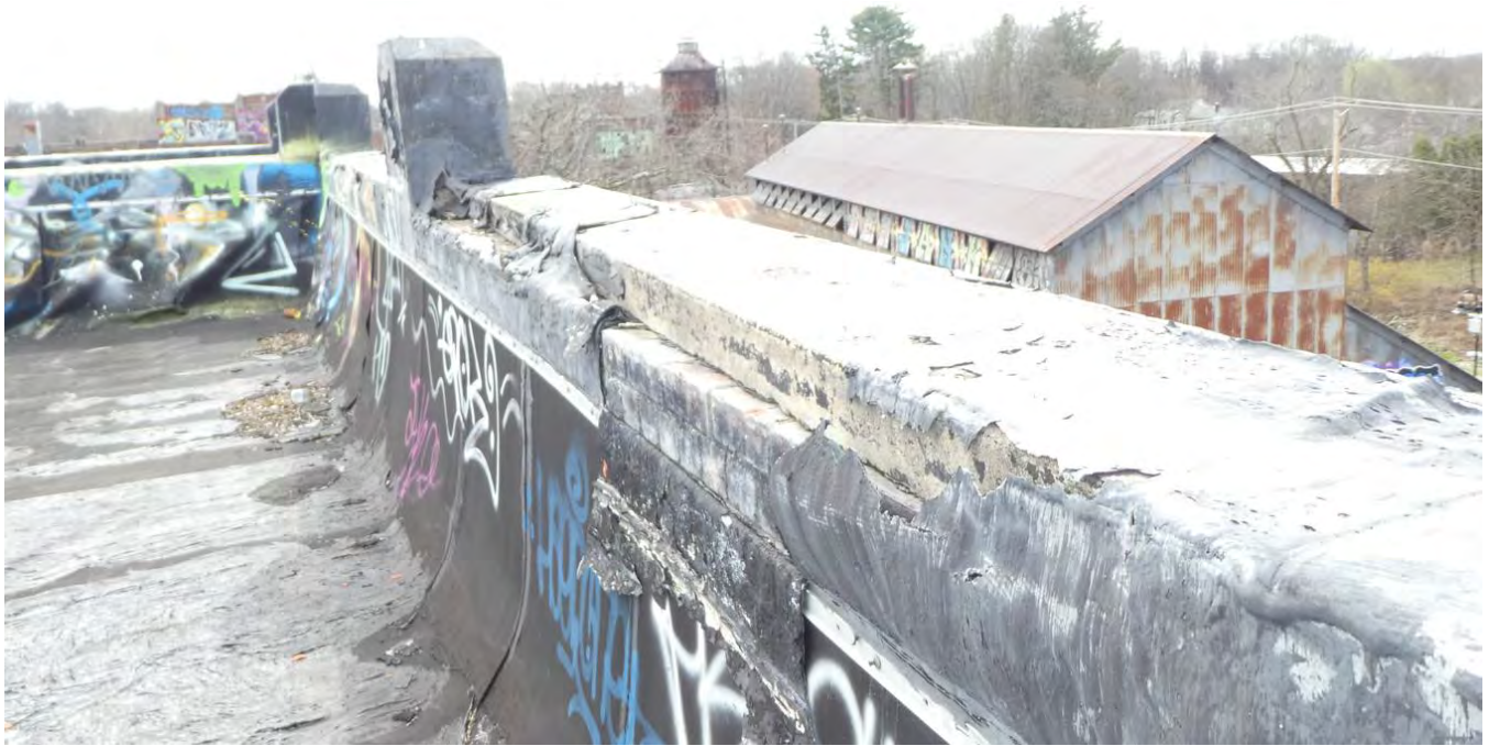
Photo 47: Building 1, west wall; coping stone at risk of falling onto lower roof.
