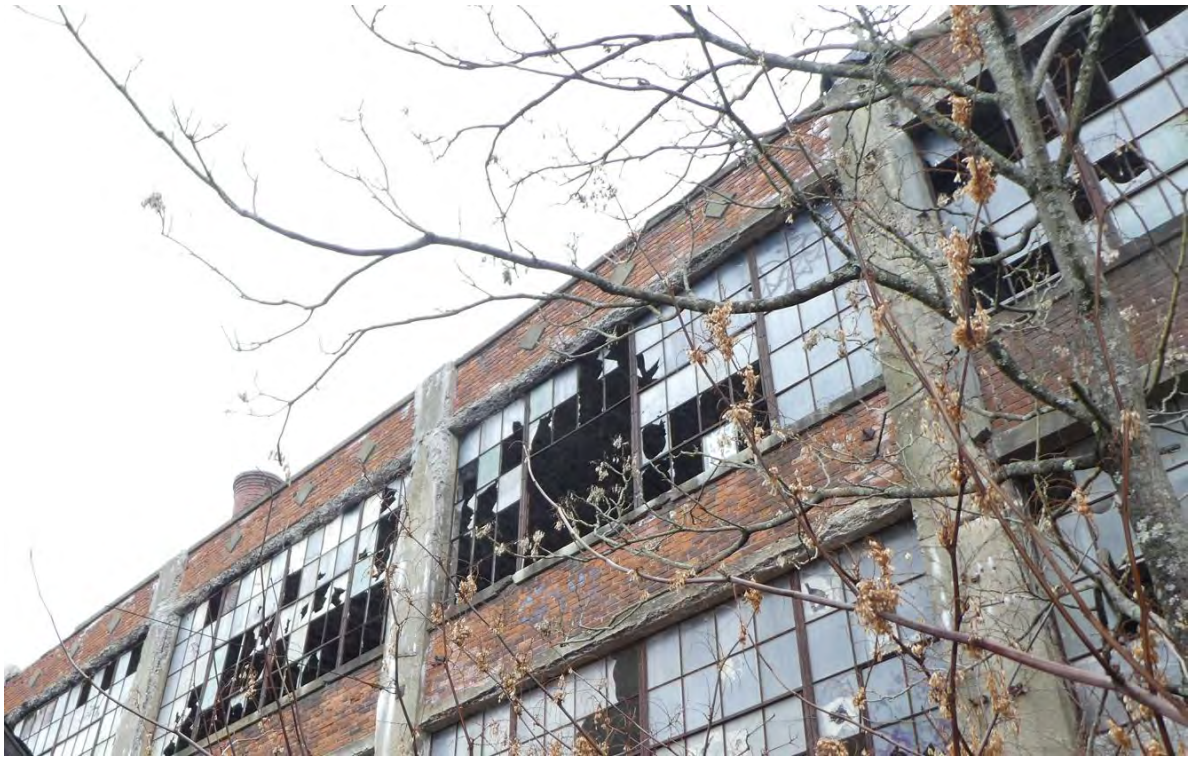
Photo 26: North Elevation Building 10, Third Floor. Deteriorated concrete columns, lintels, copings.
