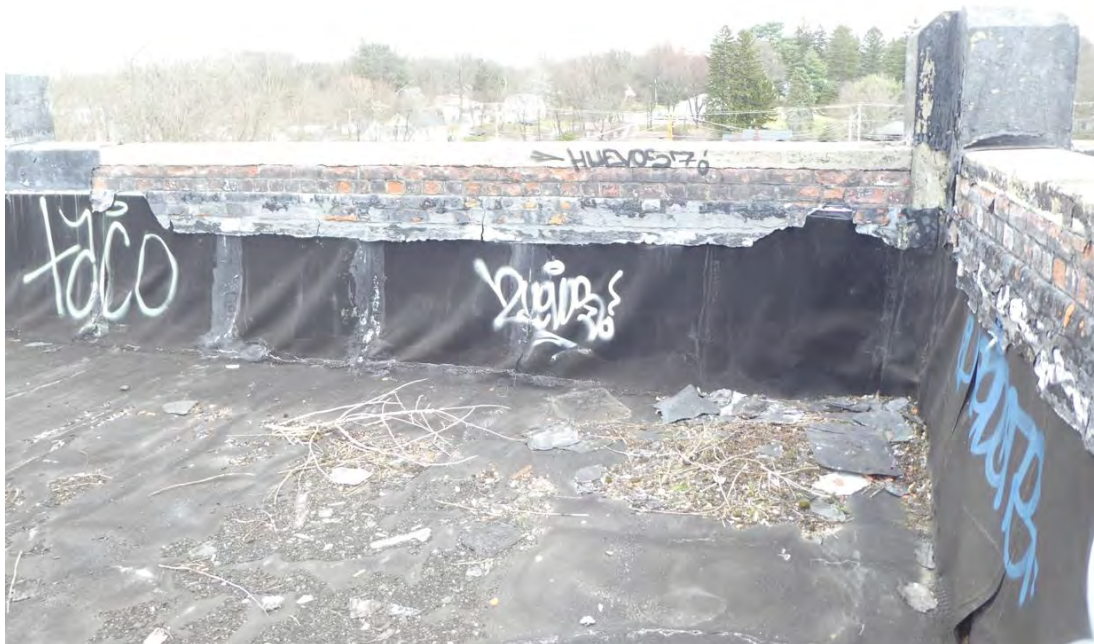
Photo 31: Building 1, existing membrane roof with open seams and pulled back from existing parapet.
