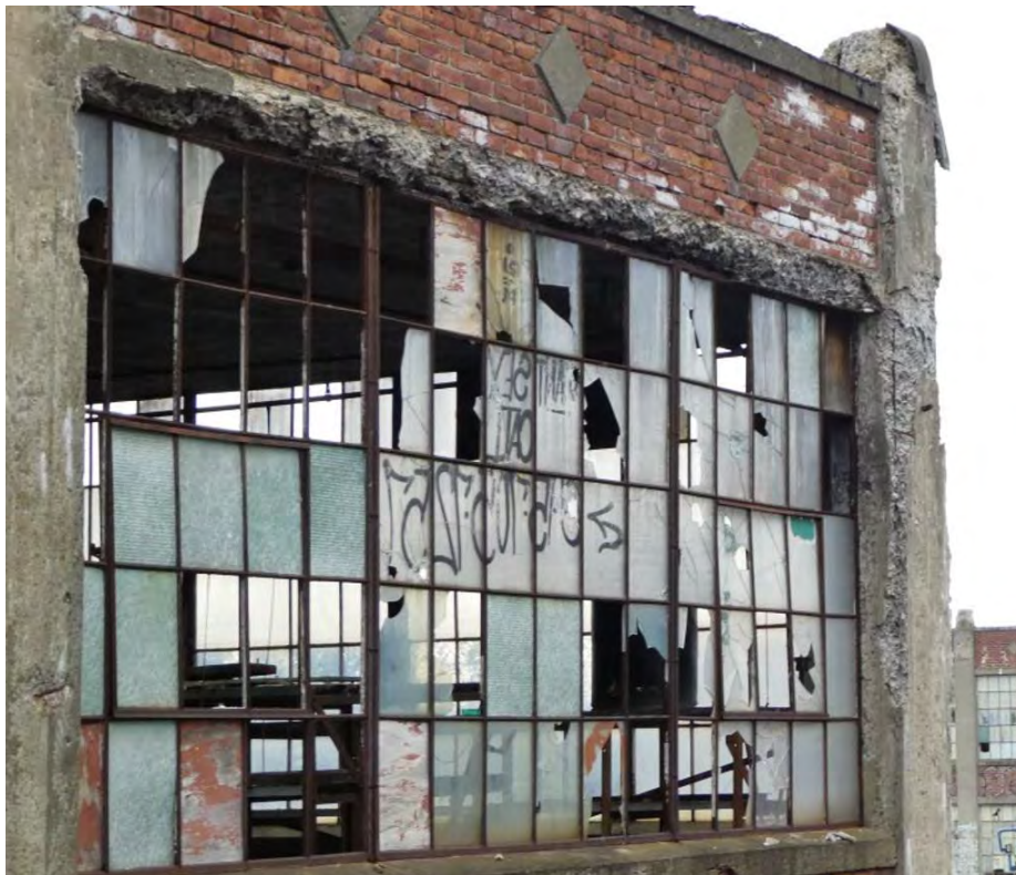
Photo 27: East Elevation Building 10, Third Floor. Deteriorated concrete columns, lintels, copings.
