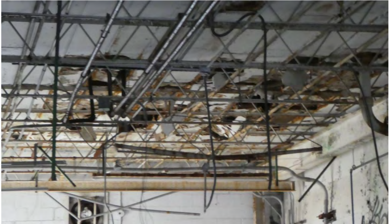
Photo 38: Building 21, gypsum plank deck failure.
