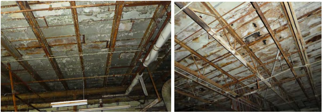
Photo 42 (left): Typical structural steel spandrel beam corrosion (Building 8); Photo 43 (right): Typical open web metal joist corrosion (Building 21).
