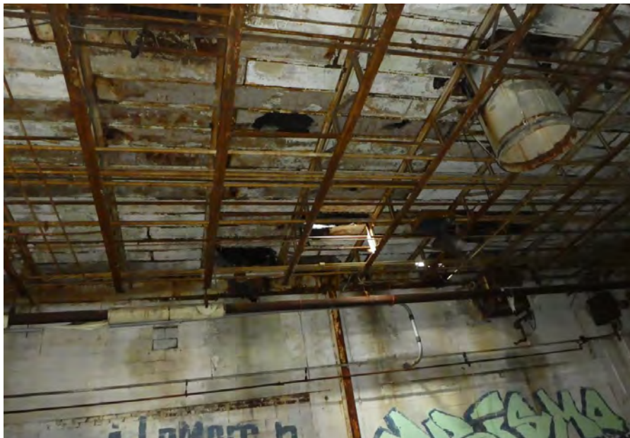
Photo 33: Building 3, gypsum plank deck failure.
