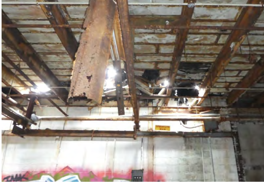
Photo 32: Building 2, gypsum plank deck failure.
