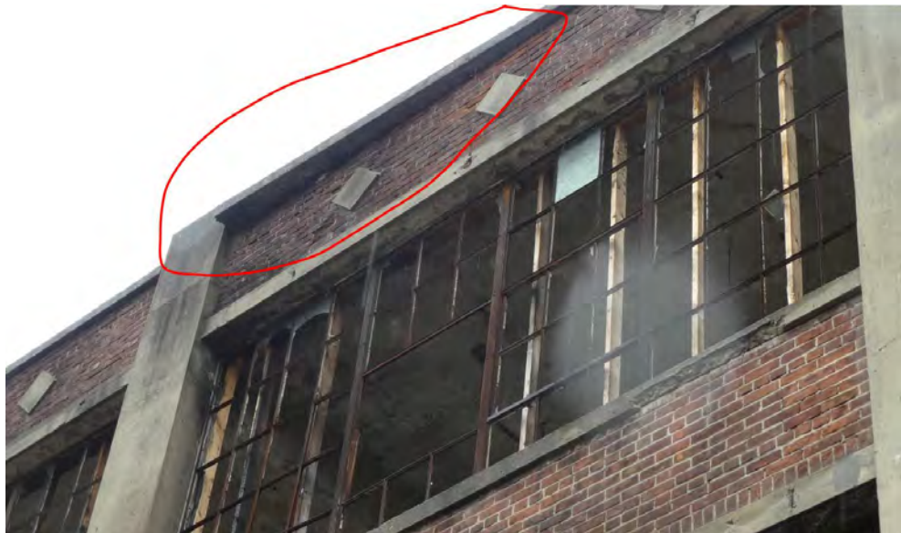
Photo 62: Building 14 parapet coping stone loose.
