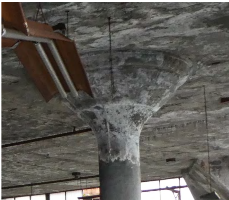
Photo 41: Typical concrete deck with calthemite straw stalactites along ceilings.
