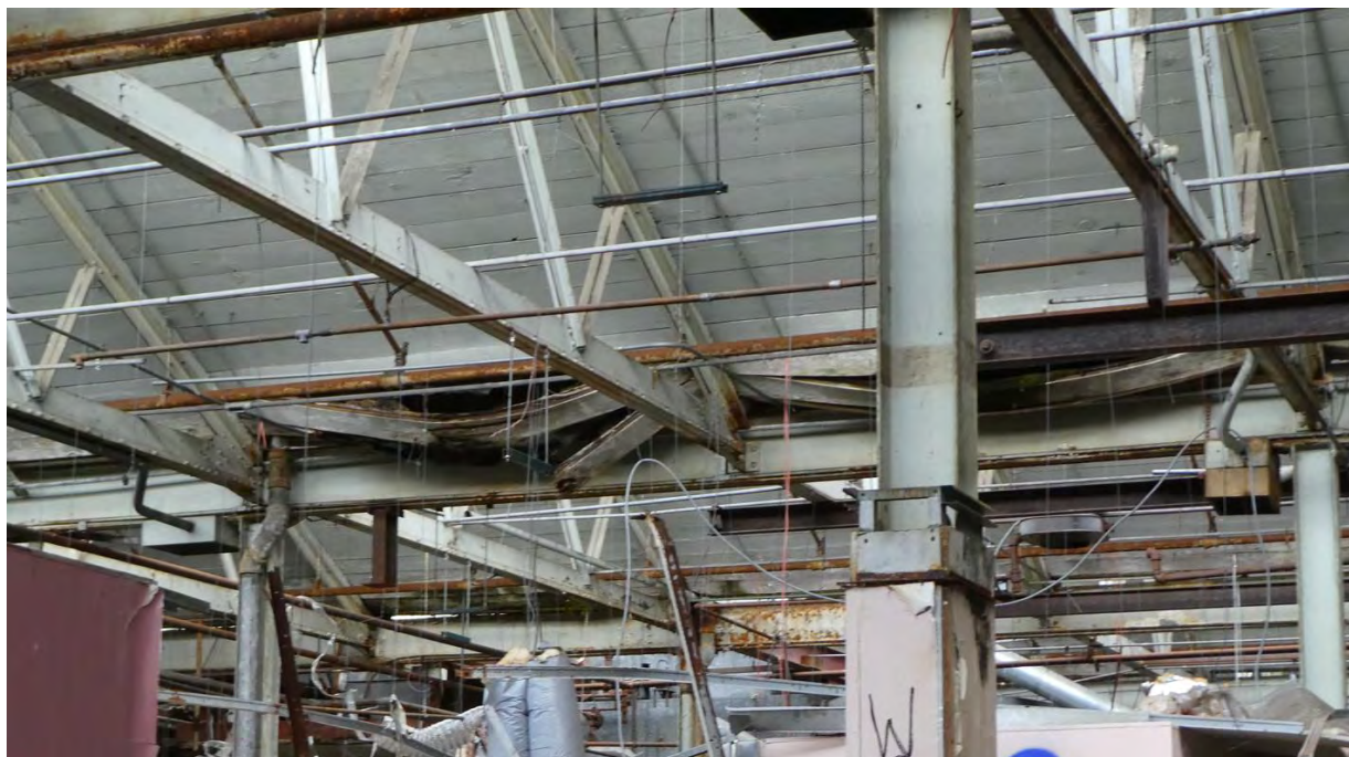
Photo 34: Building 4, wood plank deck failure.
