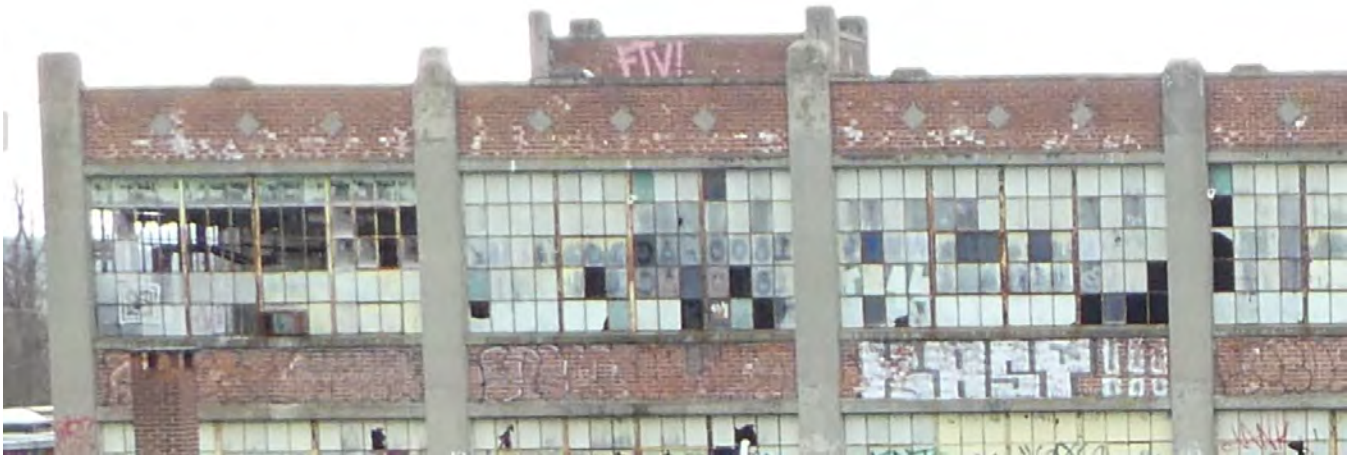
Photo 24: South elevation of Building 1. Deteriorated concrete lintels, columns, column capitals and parapet copings.
