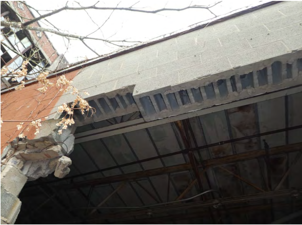
Photo 61: Building 7, brick fragments and deterioration along base of wall.
