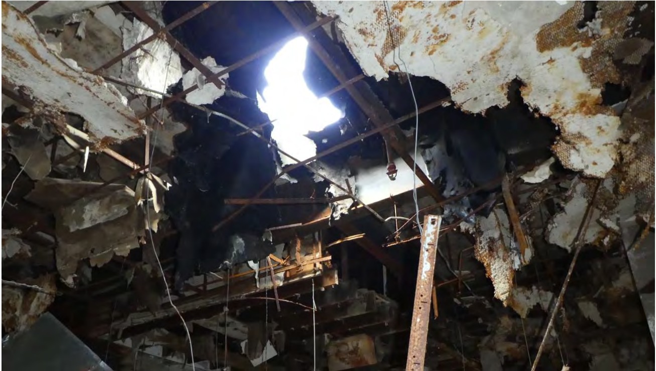
Photo 36: Building 6, poured gypsum deck failure.
