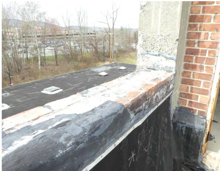
Photo 44: Building 1, west wall missing roof parapet coping stone.
