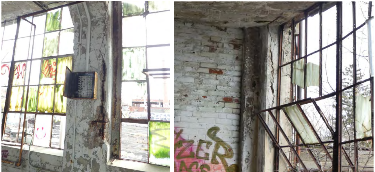
Photos 50 and 51: Building 1, cracks and exposed reinforcing in exterior concrete columns.
