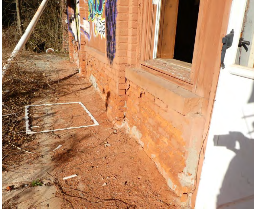
Photo 52: Building 7, brick fragments and deterioration along base of wall.
