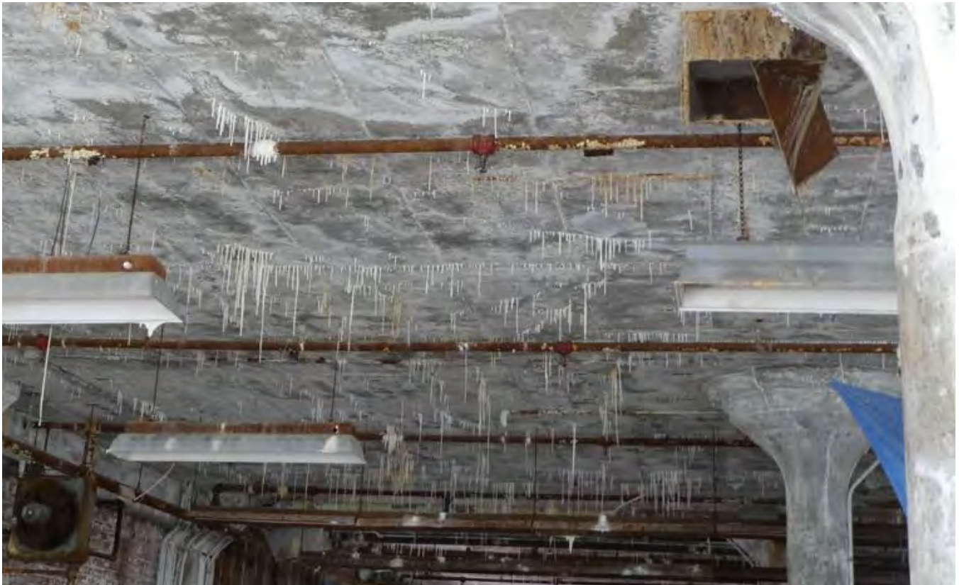
Photo 40: Typical concrete deck with calthemite straw stalactites along ceilings.
