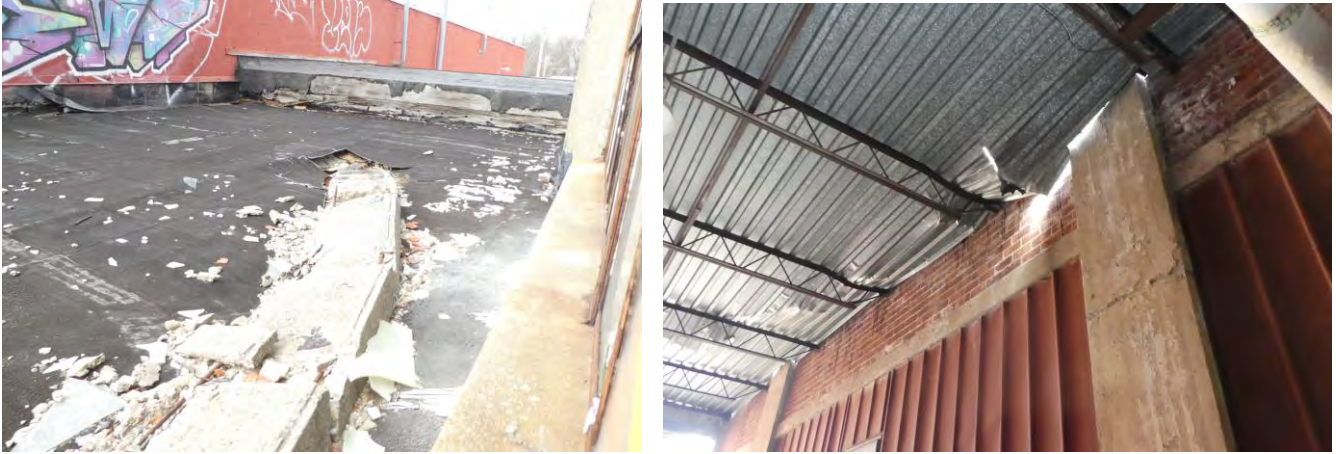
Photos 45 and 46: Lower roof west of Building 1, images of fallen coping stone and structural damage to roof deck and joists.
