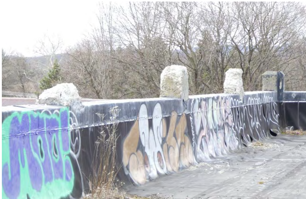
Photo 25: Building 1 South parapet wall; deteriorated column capitals.
