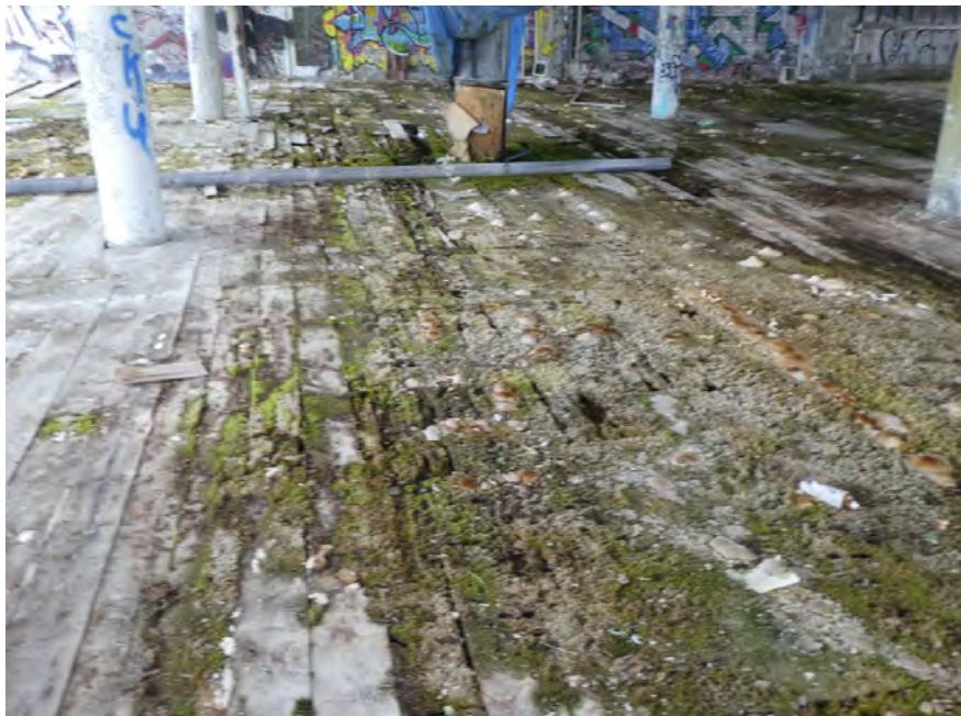
Photo 39: Typical concrete deck with wood plank flooring; organic growth.
