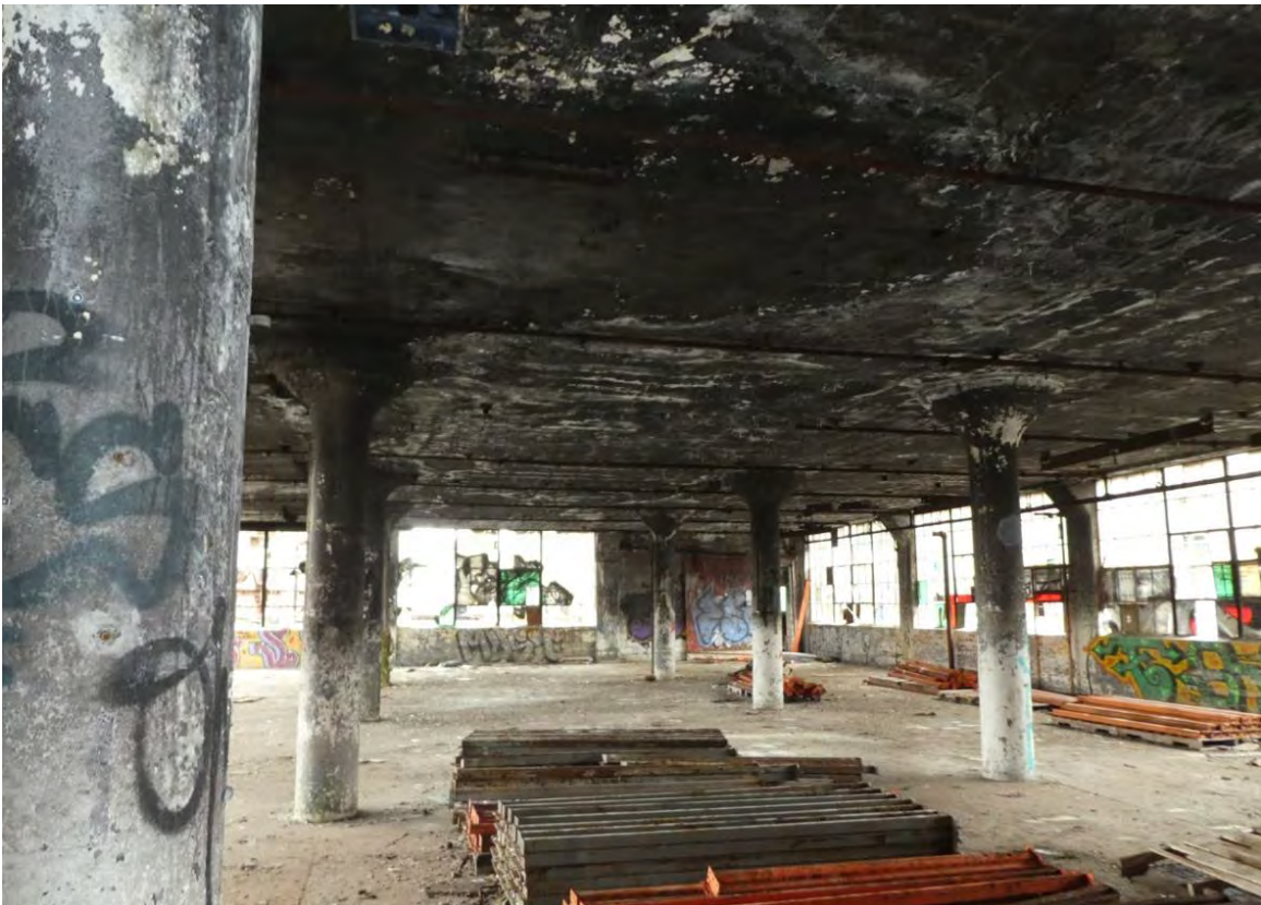
Photos 55 (above): Building 14 second floor, staining from fire damage (looking north) and Photo 56 (below): Building 12 second floor, staining from fire damage (looking north).
