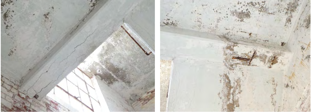
Photos 48 and 49: cracked 3 rd floor landing beam and exposed, corroded reinforcing bar.
