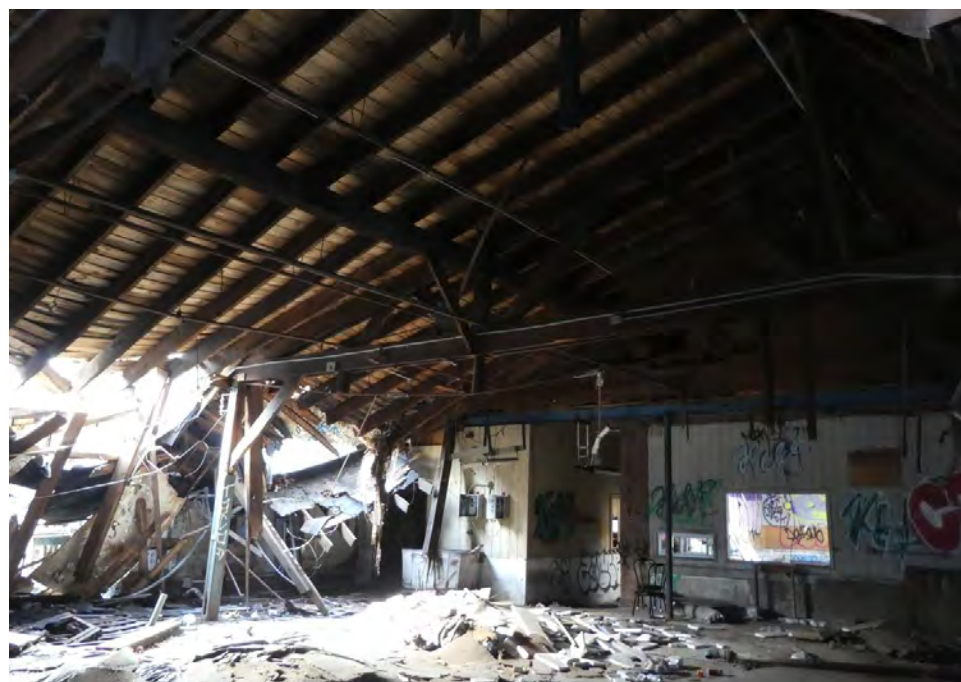
Photo 16: Partially collapsed timber building, looking southwest from building 18.
