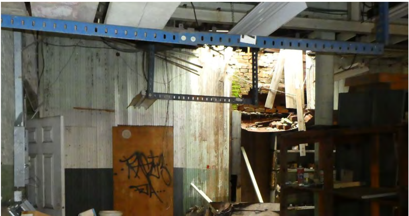
Photo 37: Building 7, wood plank deck failure.
