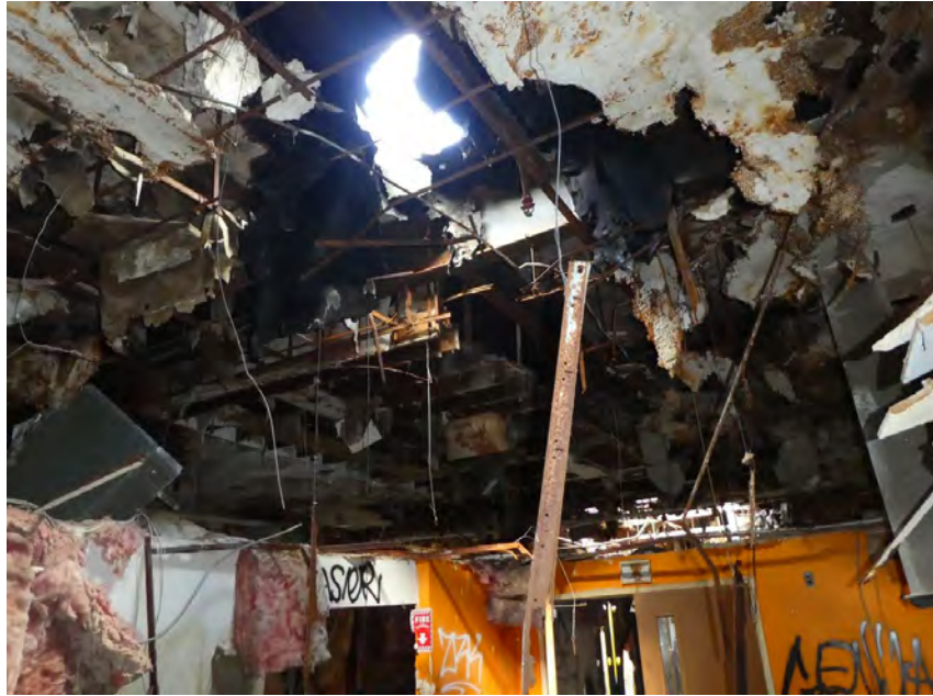
Photo 6: Building 6, looking north up at collapsed roof.
