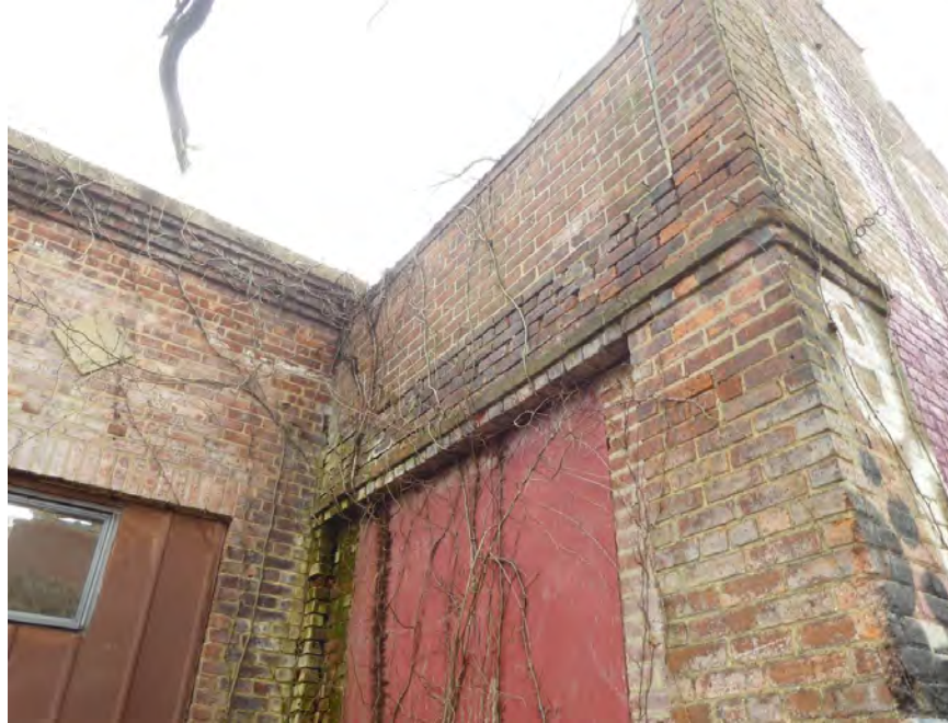
Photo 28: North Elevation Building 9. Typical occurrence of organic staining (algae, vines) and graffiti.
