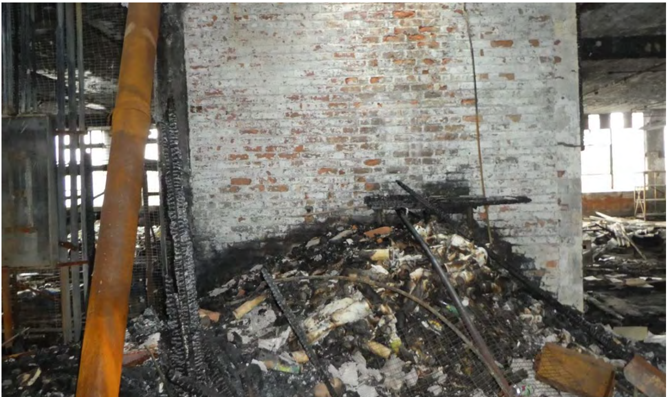
Photos 57 (above): Building 10 third floor, staining from fire damage (looking northeast) and Photo 58 (below): Building 10 third floor, building debris from fire at freight elevator (looking north).
