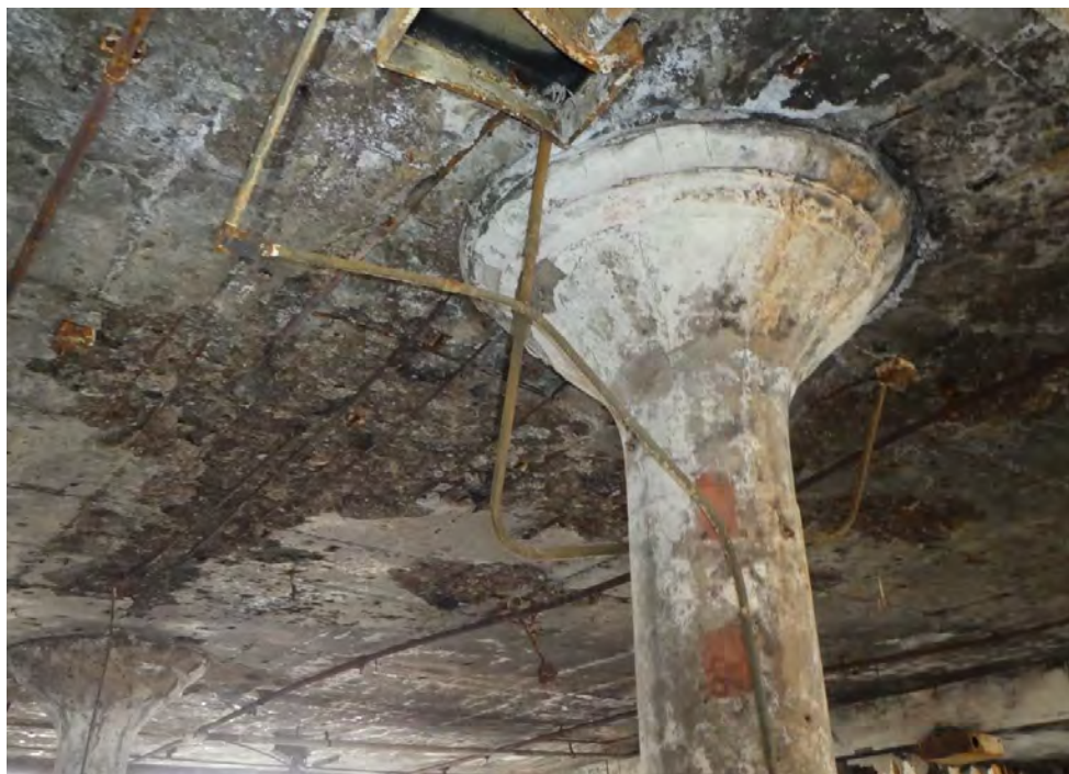
Photos 59 (above): Building 12 third floor, concentrated stored materials (looking southwest) and Photo 60 (below): Building 12 second floor looking at third floor bottom of slab, spalling, exposed rebar and sagging of slab under stored materials (looking southeast).
